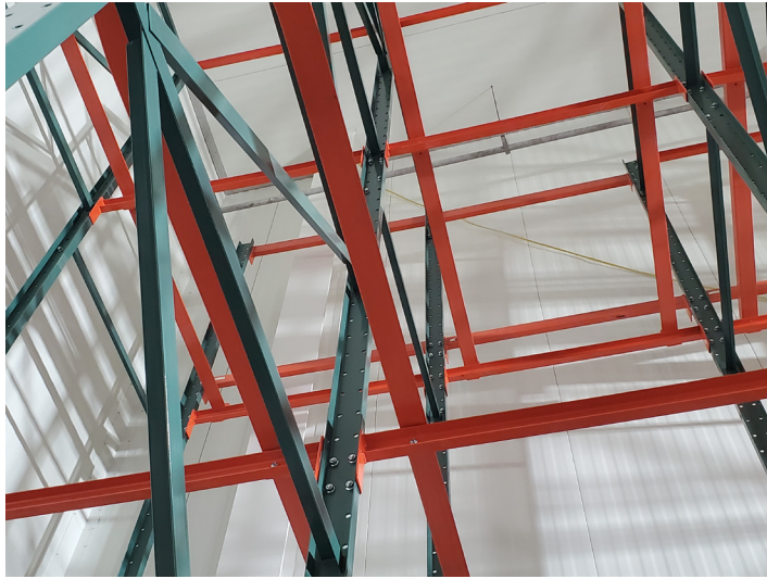
Structural Drive-in Racking Utilized in Tempering Area
